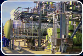
Reaction Furnace Waste Heat Boiler
